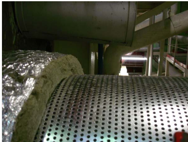
Fig. 2. A pipe insulated with noise-reducing materials
