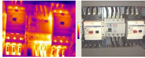
Figure 3. Thermography of panels fuses [3]
