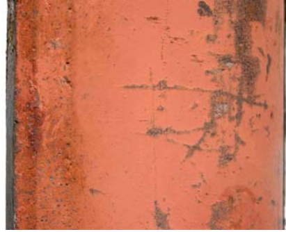
Figure 5 Tube insulation side outer surface
