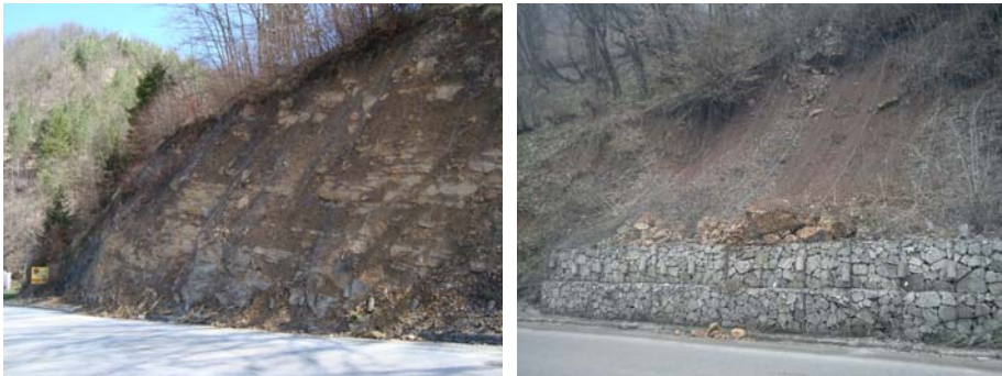
Figure 1. The inefficiency of measures of protection on the slopes (Photo: A. Ibrahimović, 2010/2011)
