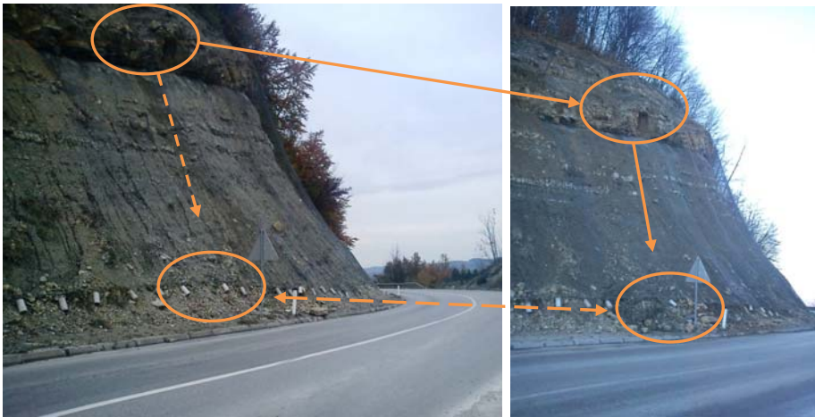
Figure 2. Monitoring of slope in the function of selection of the optimal geotechnical protective measures (Photo: A. Ibrahimović, 2010/2011)
