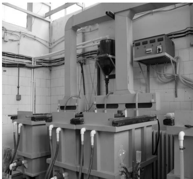
Figure 1. New pilot plant for electrolytic refinig copper-Line 1
