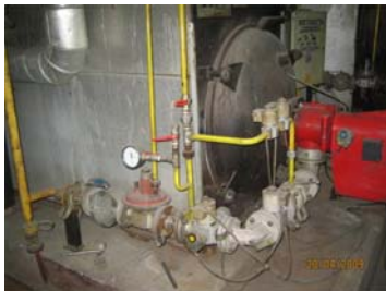
Figure 4. View on the old boiler
