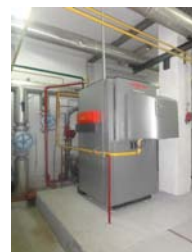
Figure 5. View on the new condensing boiler
