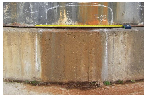
Corrosion products as sign of bottom perforation
